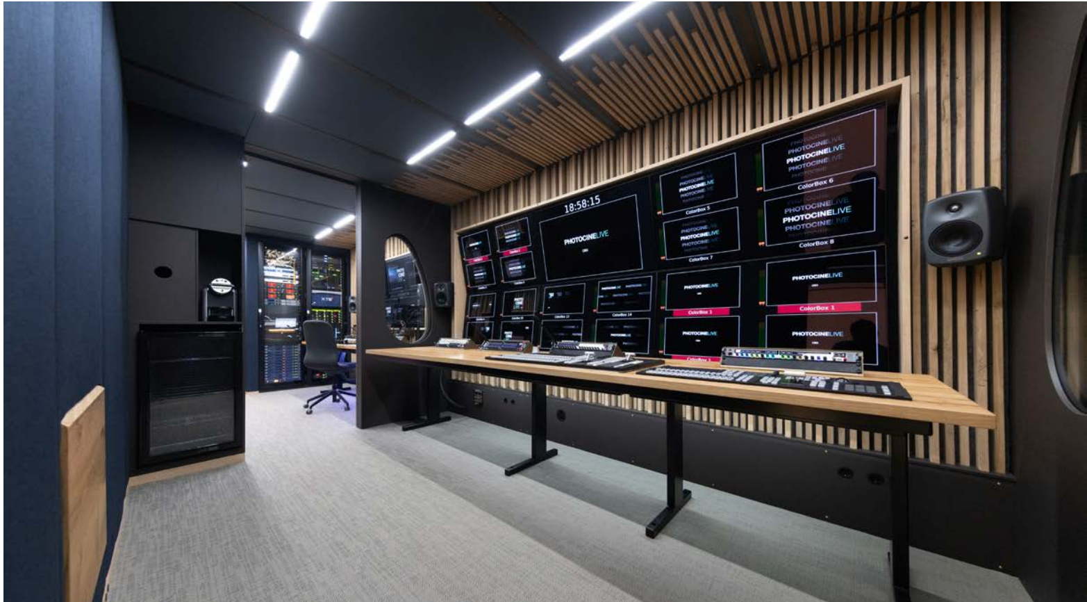
Production area: Sony XVS G1 UHD switcher 24 In / 12 Out, ICP-X1224 & X1116 panels. 6x LG 48" HDR OLED monitors. Ross FR12 Router. Riedel Artist 1024 intercom system with 1200 series panels and Bolero Beltpacks. Refrigerator. Nespresso coffee machine. Separate Audio Room with Yamaha DM7-EX console, Genelec 5.1, DANTE network, Netgear AV Switches.
